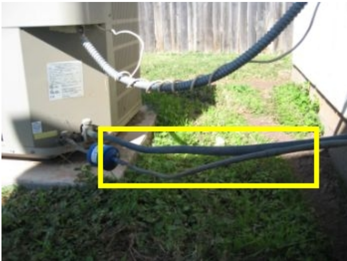
Refrigerant lines are missing insulation in areas
