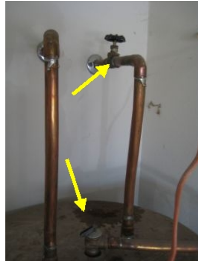
Evidence of leaking was visible
