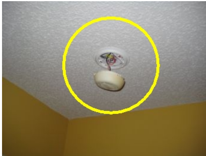
Smoke detectors are hanging from ceiling in numerous locations
