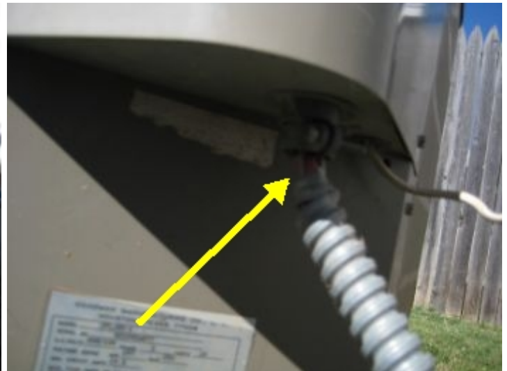
Wires going into unit not properly attached see pictures
