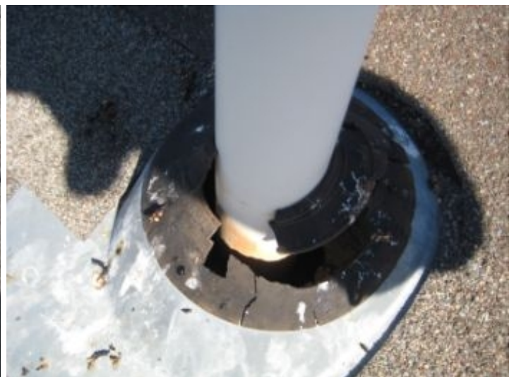
Holes present around vent(see Picture)
