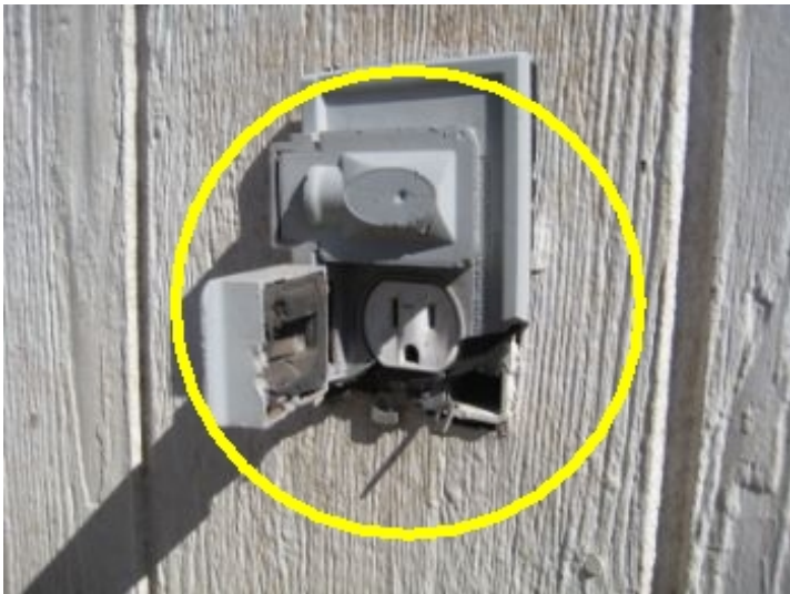
Exterior cover damaged cracked along bottom see picture/back porch
