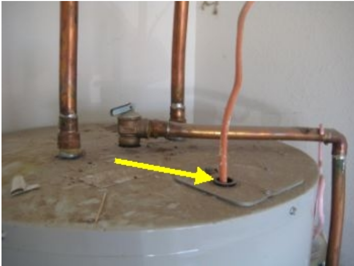
Electric source not properly connected to heater
