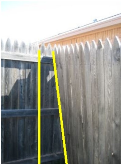
Fence leaning in back yard
