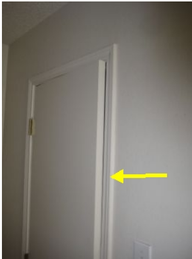
Master bedroom closet door did not close in the jamb
