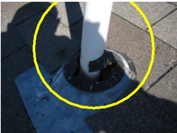
Holes present around vent(see Picture)
