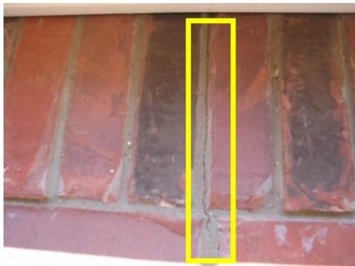
Exterior crack less then 1/8 mainly cosmetic
