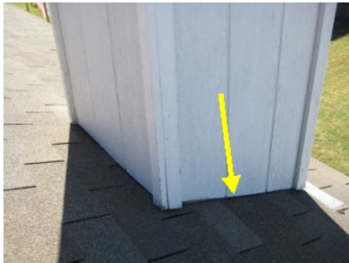
recommend step flashing around chimney
